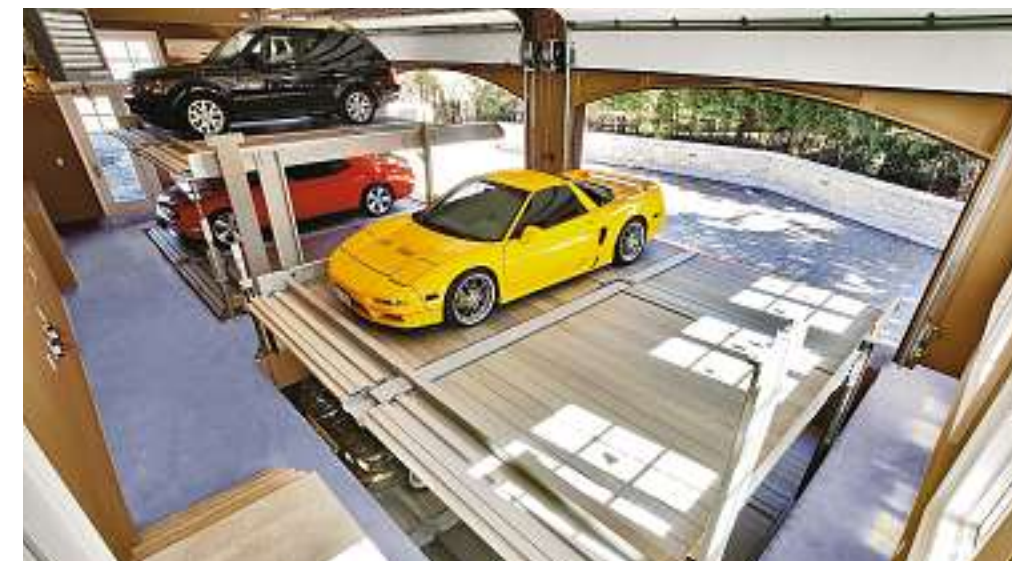
The "climatized" garage includes a European car lift system (with a capacity for eight cars), an elevator and a glycol snow melt system.
